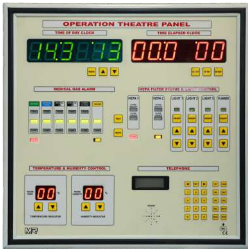
Operation Theatre Control Panel
